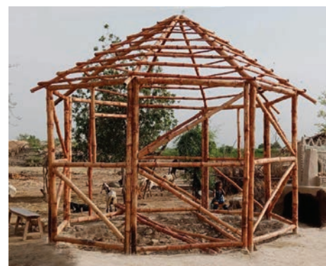
Fig. 7. Prefabricated bamboo structure of a Lari OctaGreen (LOG) one-room house, Pono Colony, Mirpurkhas, Sindh, 2022.
