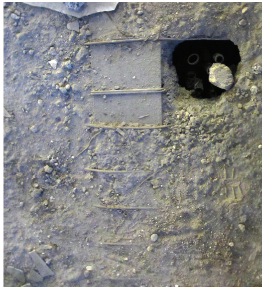
Fig. 4. Exposed mesh at the top flange of an existing beam after removal of cinder fill.
