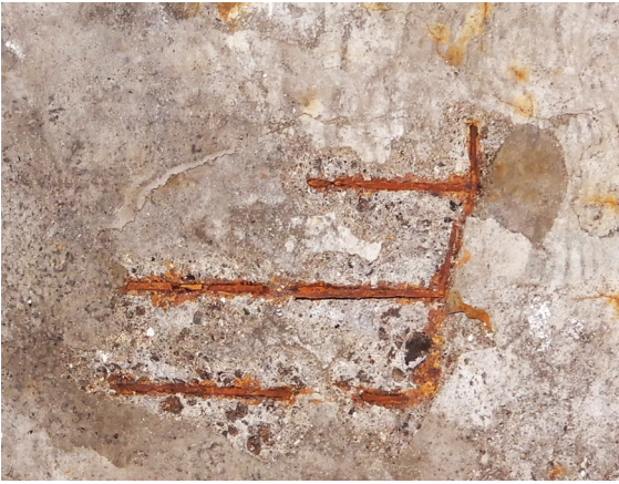
Fig. 8. Close-up view of corroded and snapped mesh at slab underside.
