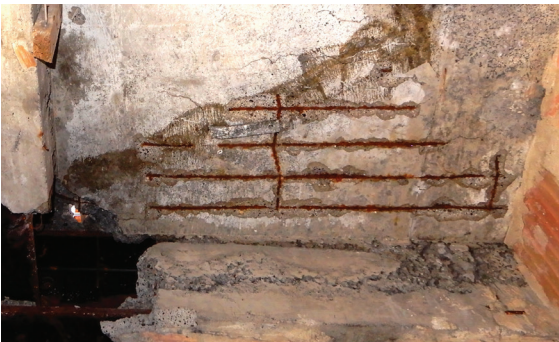
Fig. 9. Corrosion staining and complete section loss of mesh at slab underside.
