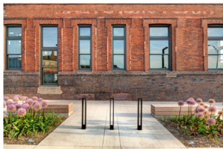
Fig. 4. Market One, north-façade windows before and after restoration. Original double-hung wood sash windows were removed, refurbished, and reinstalled. Photographs by Integrated Studio, 2015.
