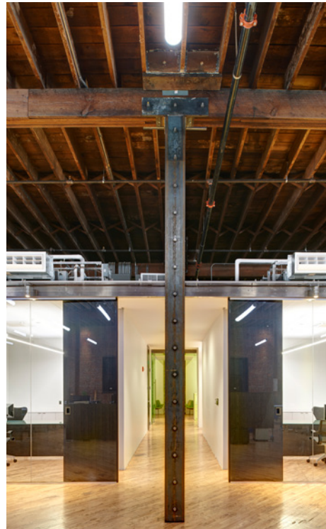
Fig. 7. Market One, interior fit-out, showing efficient mechanical systems and preserved historic volumes; the VRF system eliminated large ductwork, thereby maintaining the original spatial qualities. Photographs by Integrated Studio, 2015.
