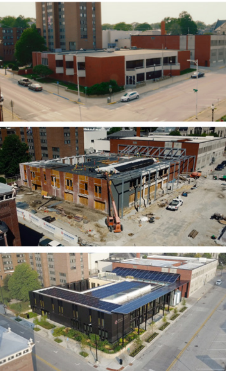
Fig. 6. Stanley Center for Peace and Security, building envelope transformation, showing the existing brick structure retained with a new thermally insulated rainscreen applied directly to minimize carbon impact. Photographs by Neumann Monson Architects, 2023.
