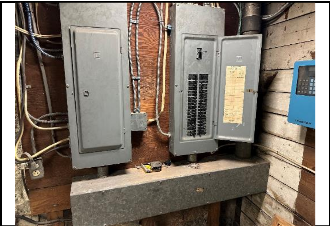
Photograph 66: Electric load centers.
