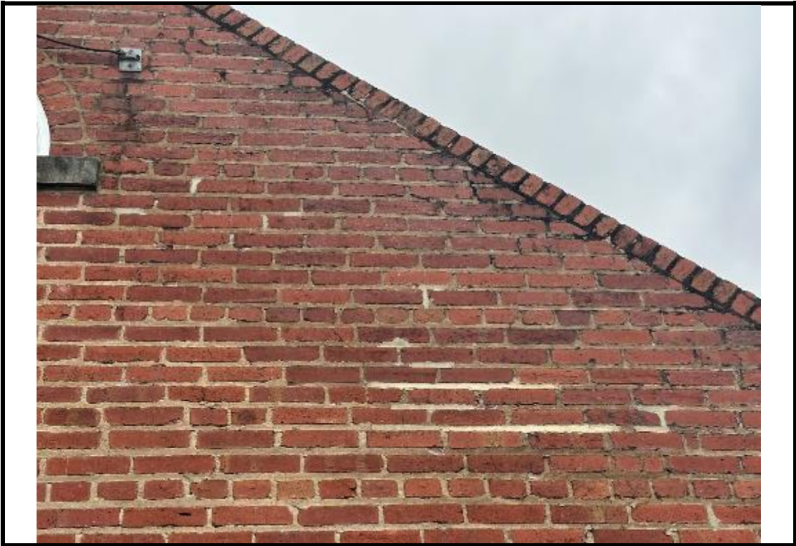
Photograph 25: Example of deteriorated masonry mortar joints.
