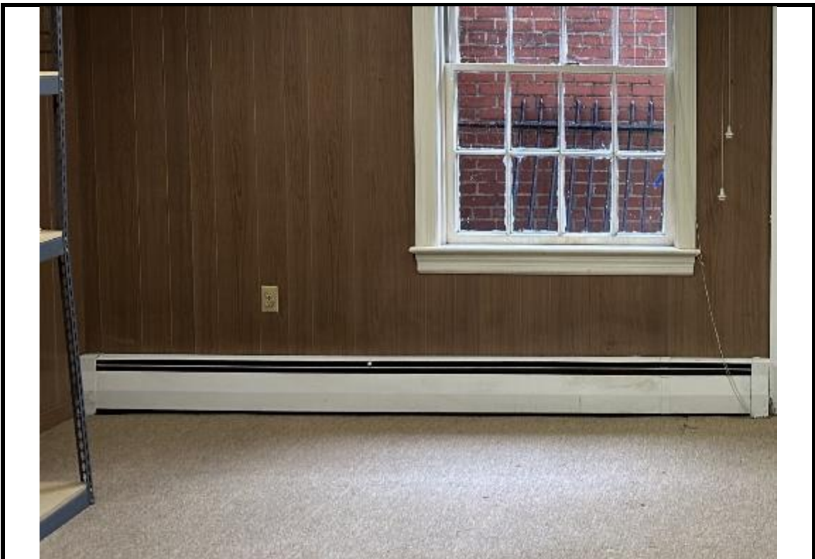
Photograph 60: Typical baseboard radiator.
