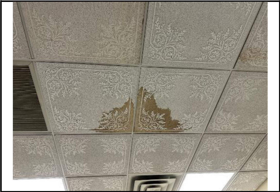
Photograph 45: Decorative suspended ceiling tiles with water stains.
