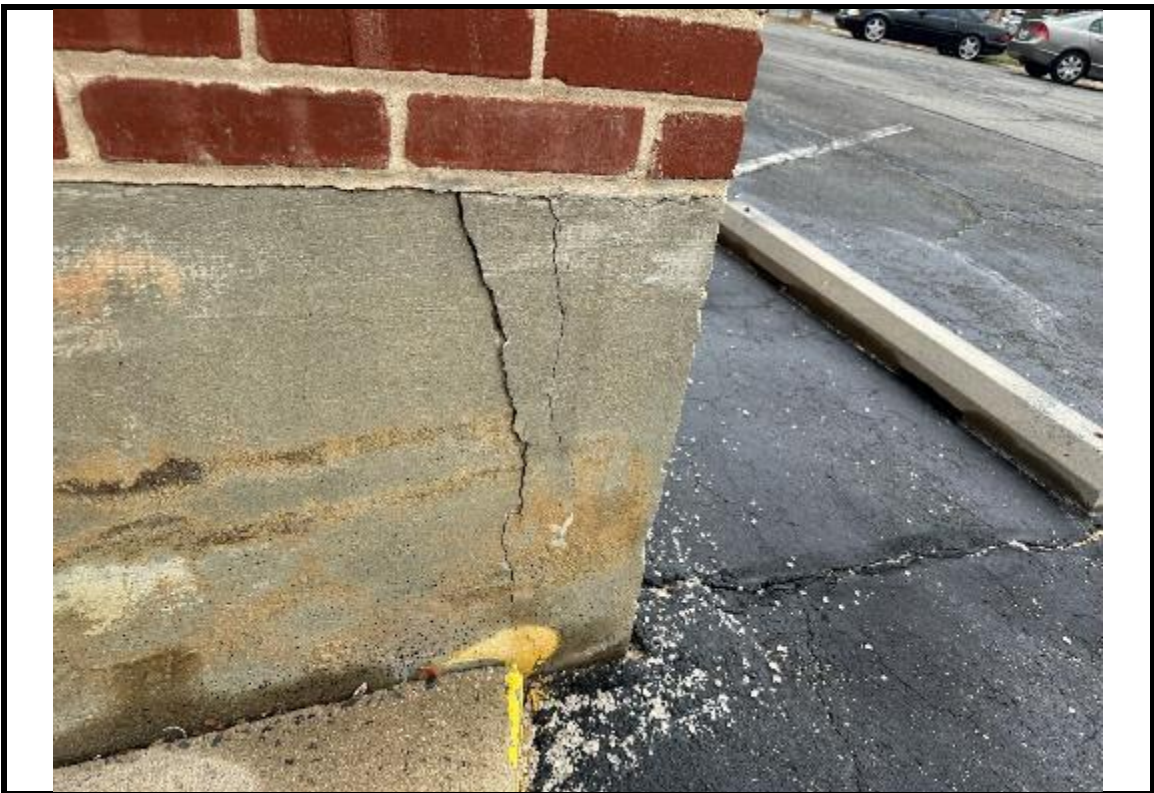
Photograph 38: Cracked foundation wall.
