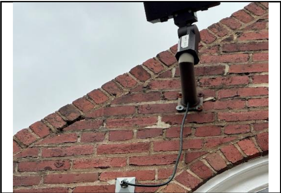
Photograph 26: Example of deteriorated masonry mortar joints.
