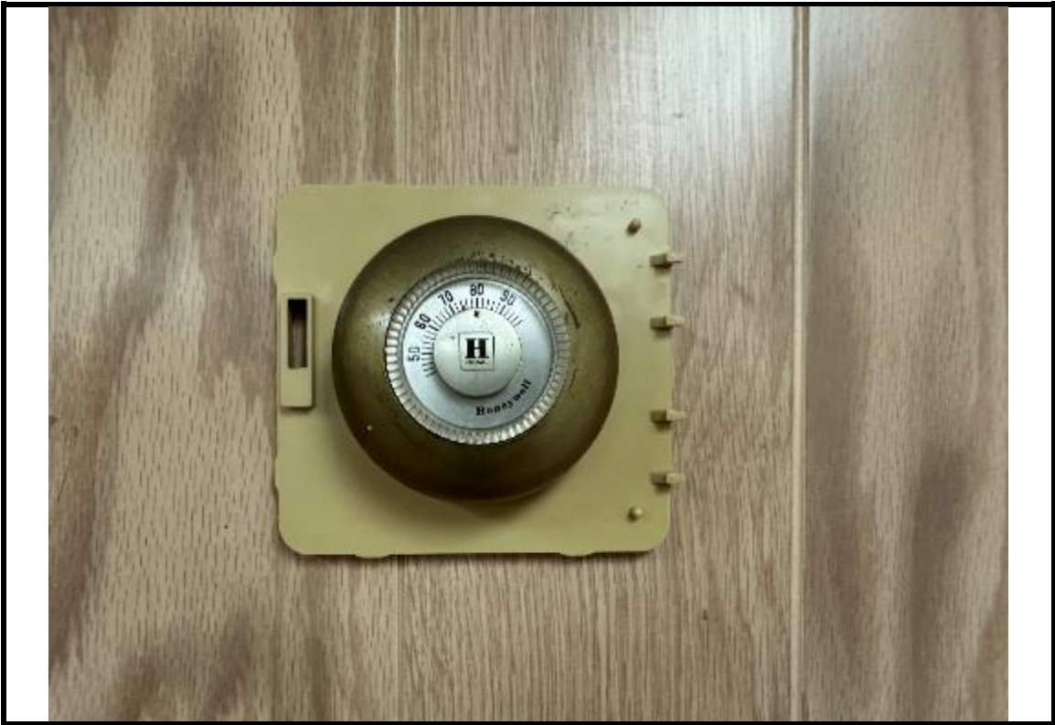
Photograph 61: Typical analog thermostat.
