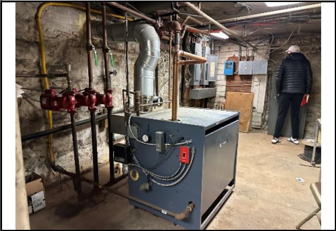
Photograph 57: Gas-fired packaged boiler.
