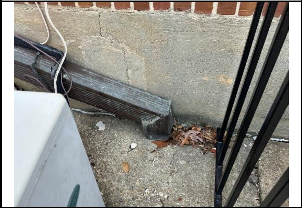
Photograph 37: Downspout in contact with the concrete sidewalk obstructing water flow.
