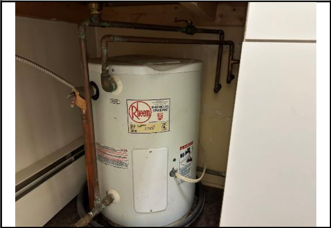
Photograph 63: Electric water heater.
