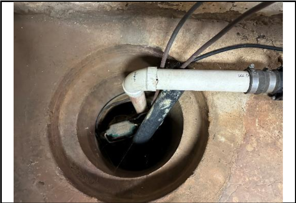
Photograph 64: Basement sump pump.
