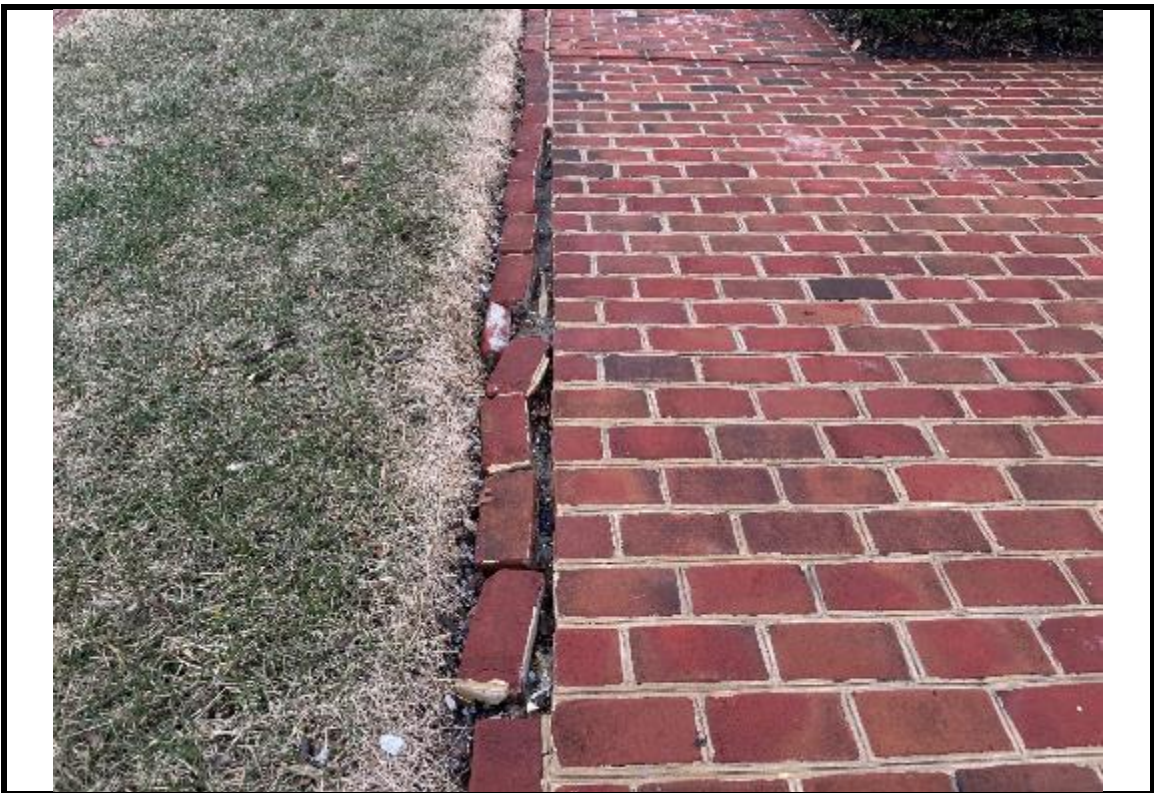
Photograph 14: Displaced pavers at the front entrance.
