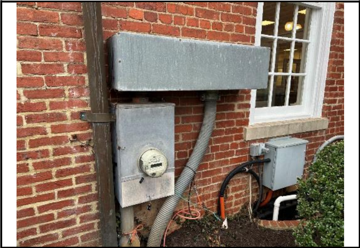
Photograph 65: Electric service meter.
