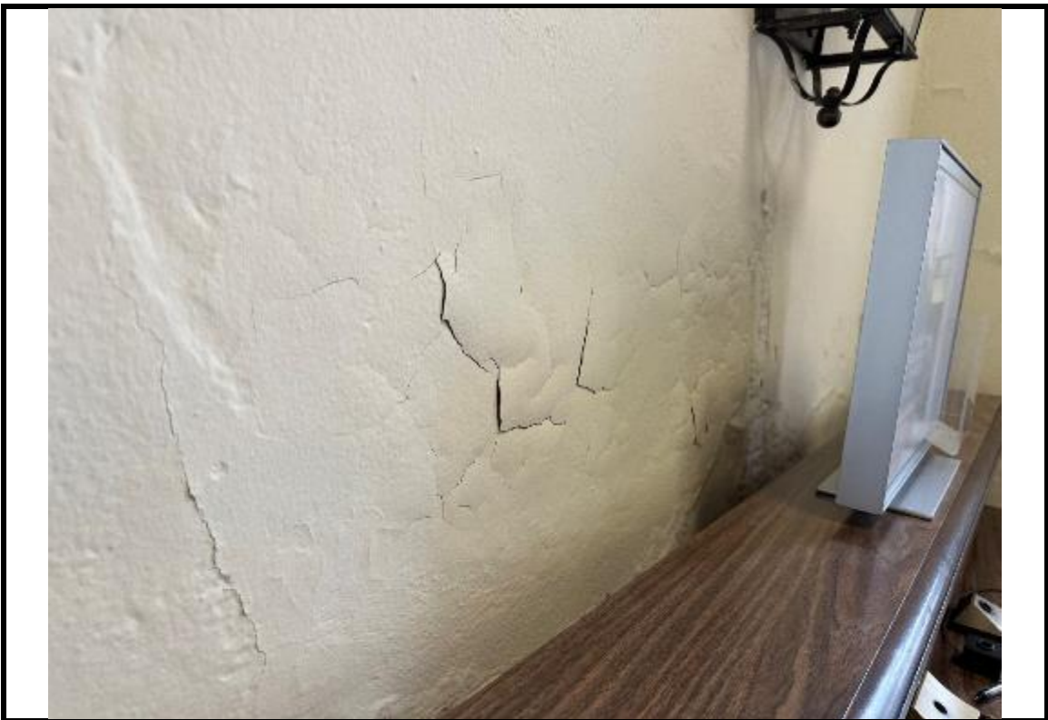
Photograph 50: Blistered plaster wall and paint.
