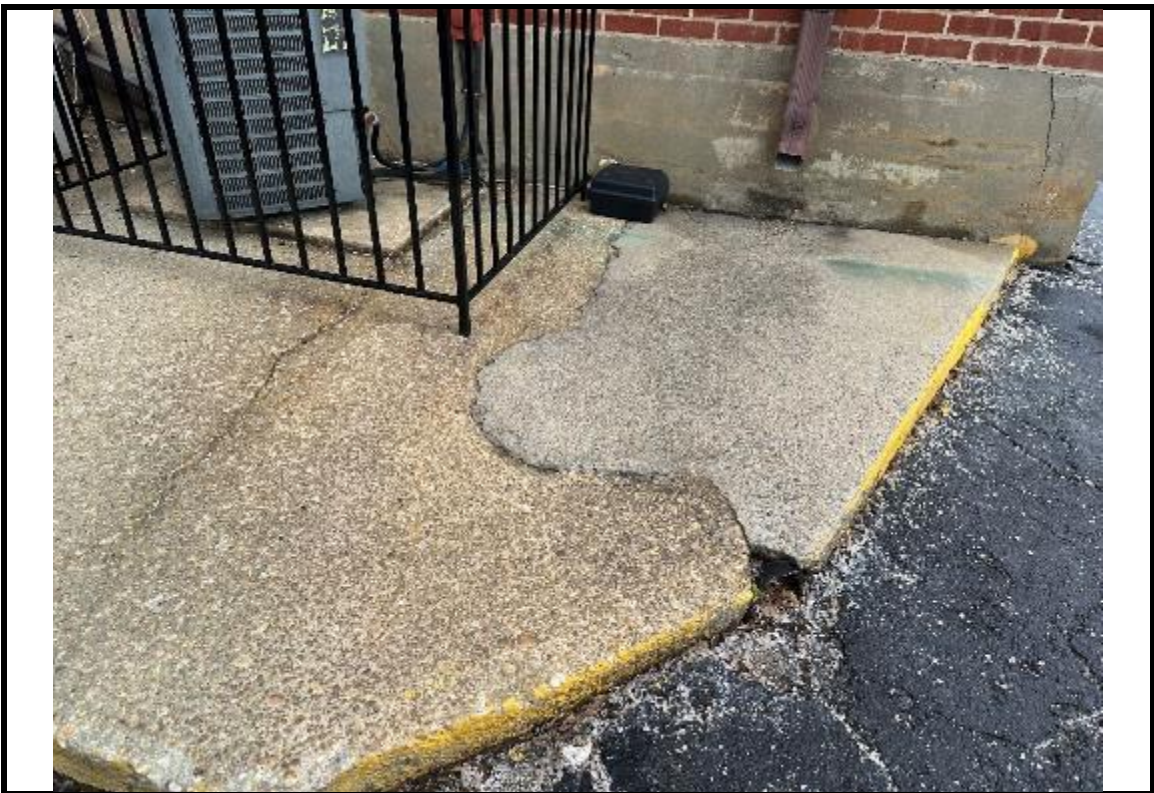
Photograph 10: Cracked concrete sidewalk.
