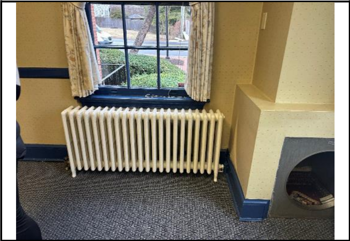
Photograph 59: Typical cast iron radiator.
