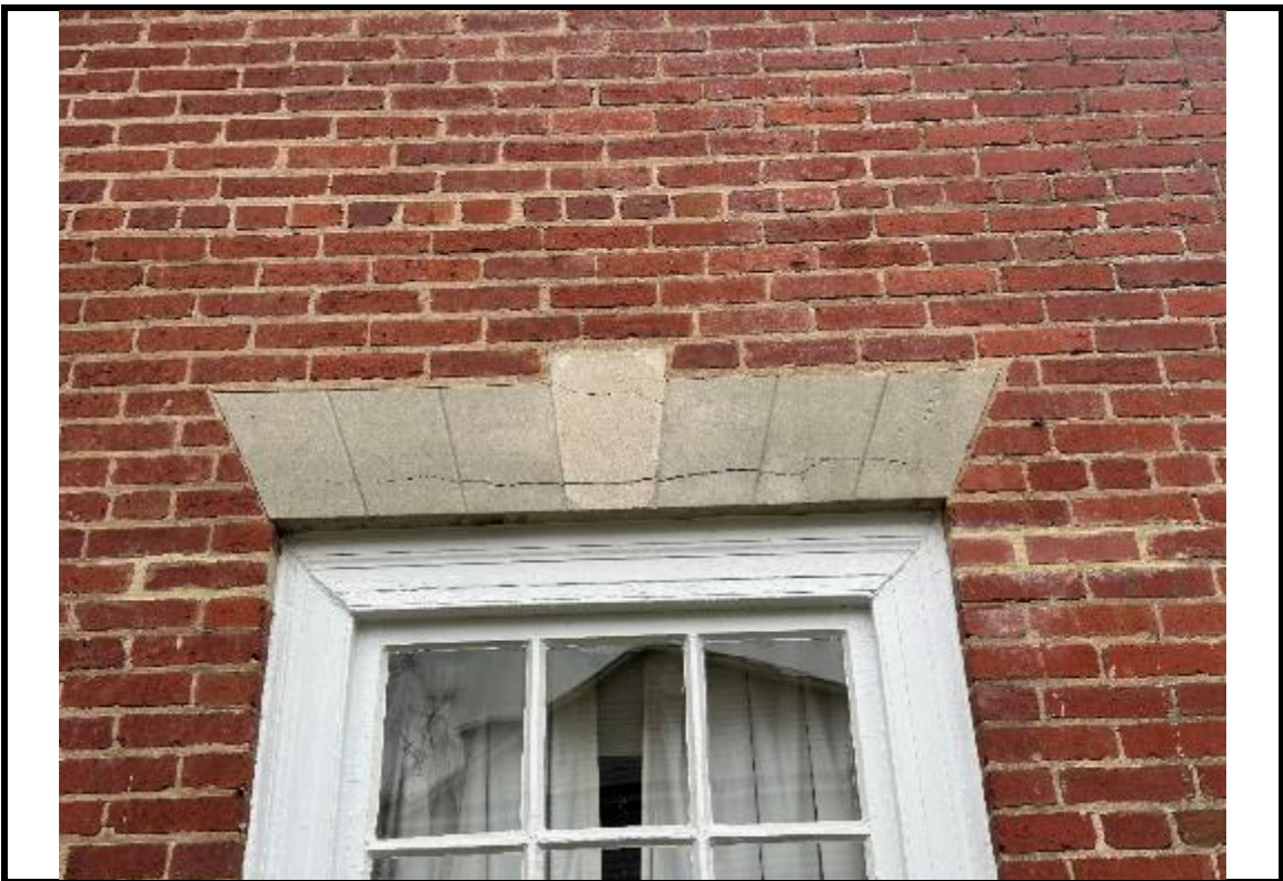
Photograph 30: Cracked cast stone above windows.
