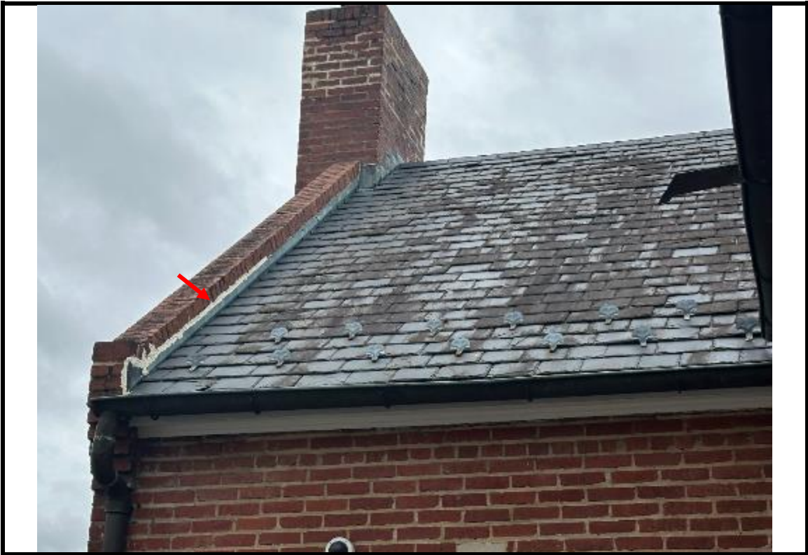
Photograph 33: Slate roof with microbial growth. Note the prior sealant repairs.
