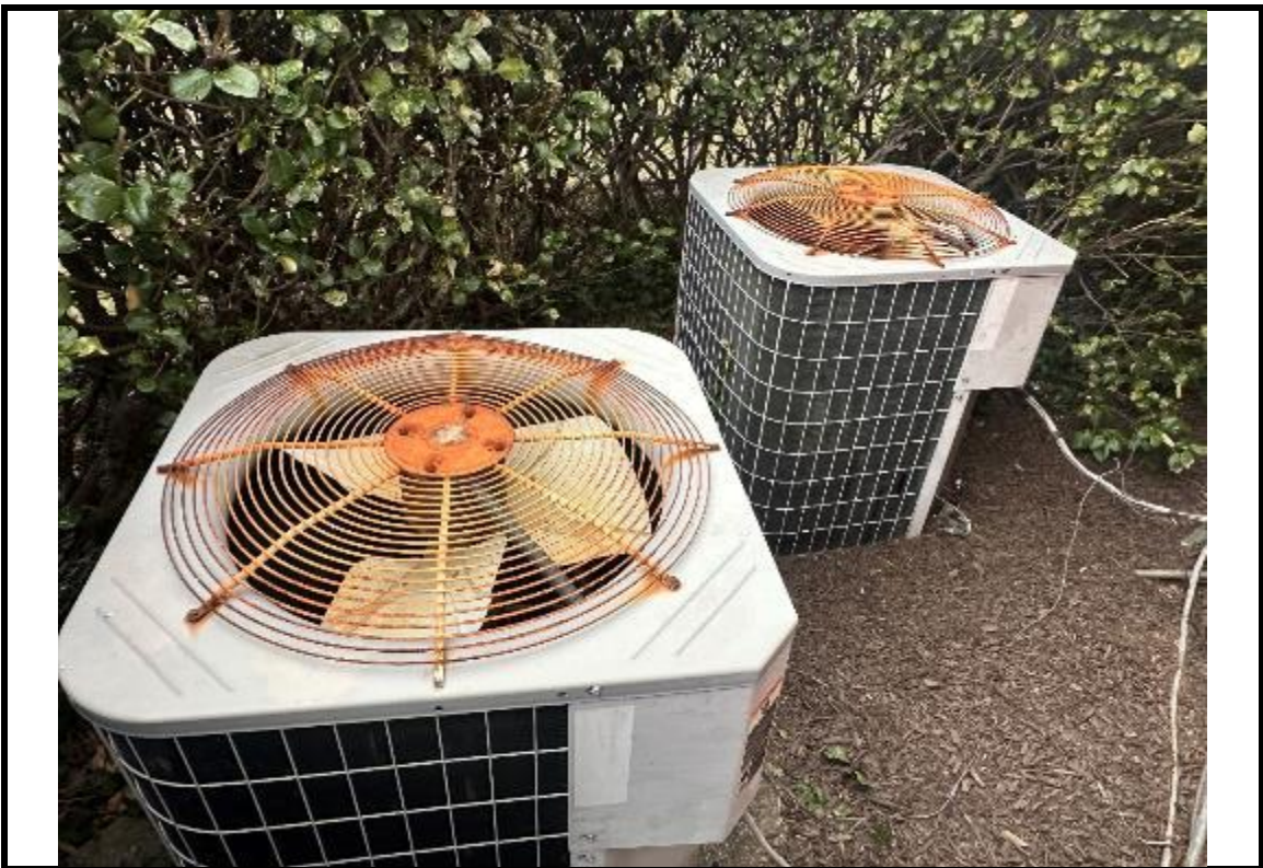
Photograph 56: Typical exterior AC condensing units.
