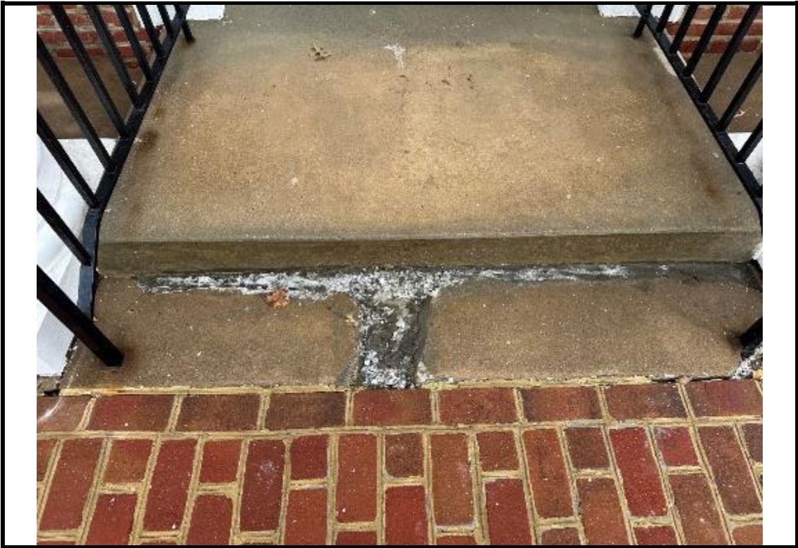
Photograph 15: Deteriorated concrete steps at the main entrance.
