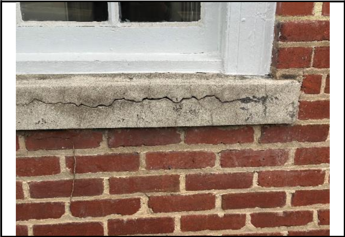
Photograph 31: Cracked stone window sill.
