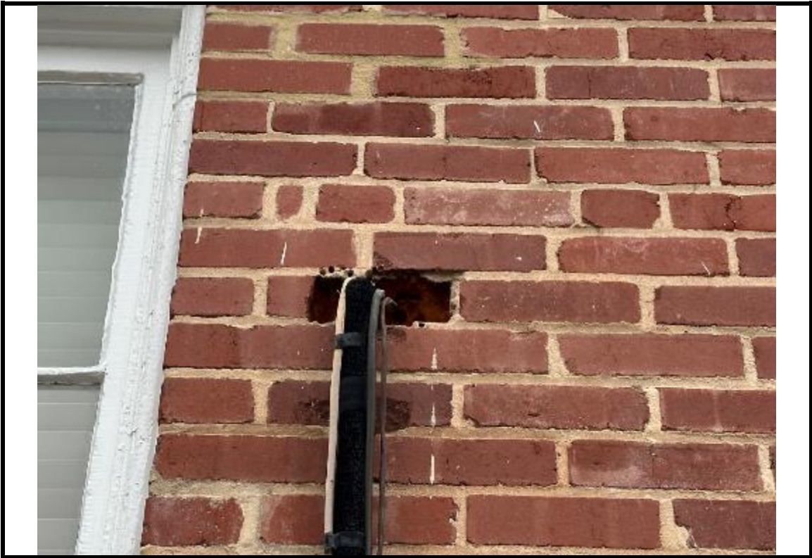
Photograph 27: HVAC line penetrations and missing brick.
