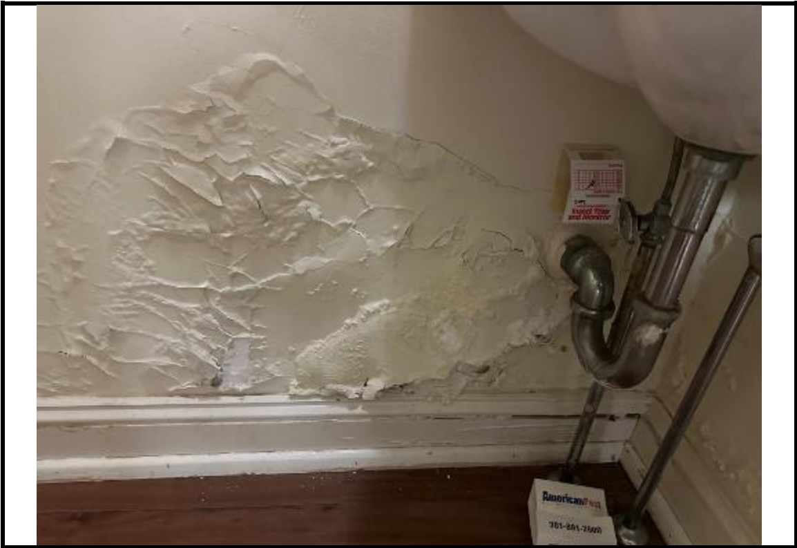
Photograph 49: Water damage on the interior plaster wall.
