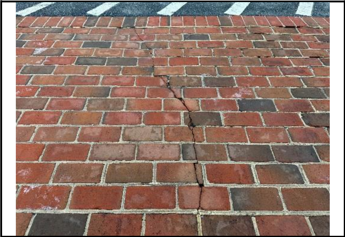
Photograph 13: Cracked paver sidewalk.
