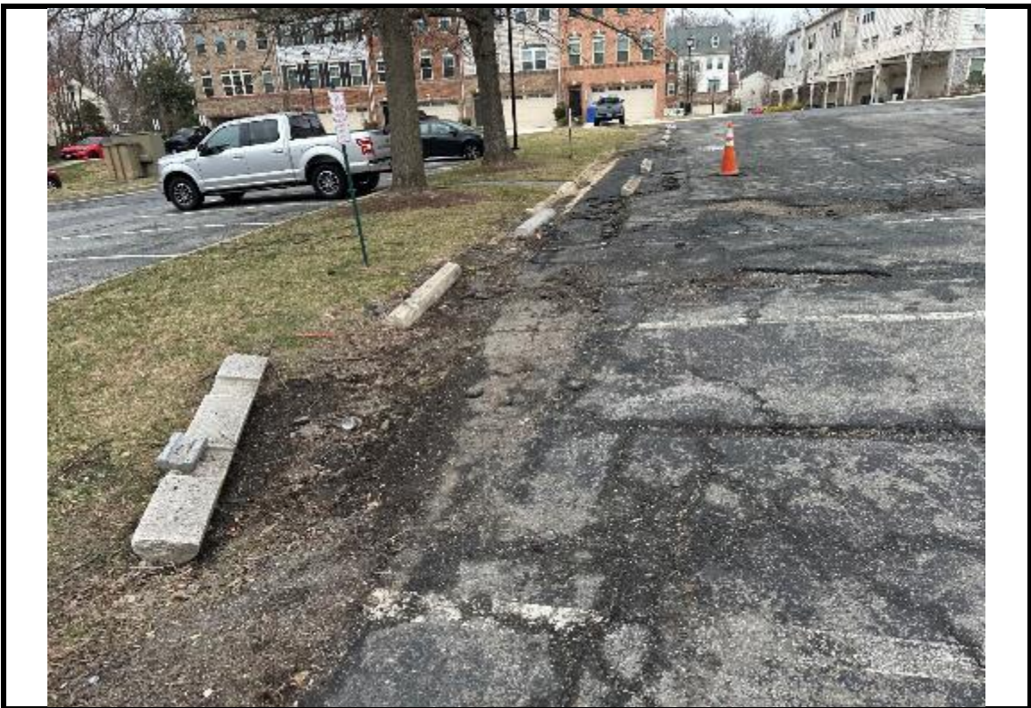
Photograph 8: Displaced wheel stops. Note the buried concrete swale.
