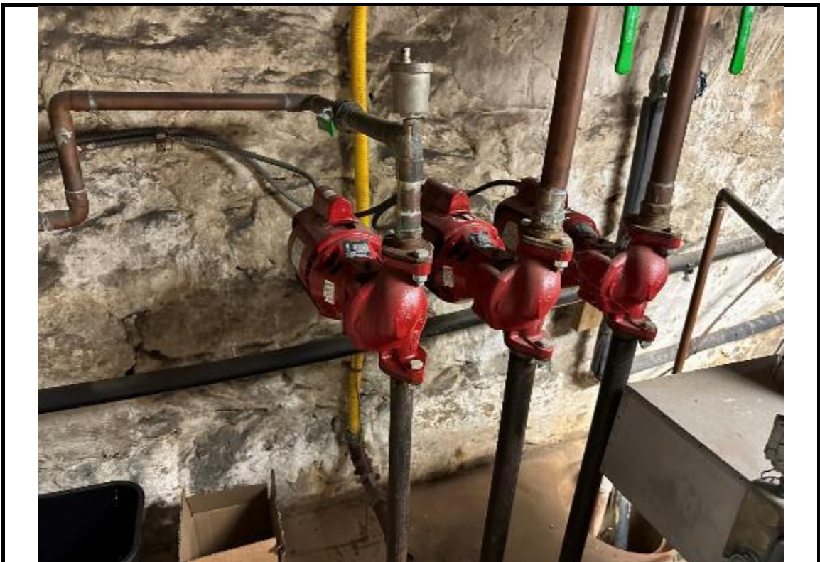
Photograph 58: Hot water recirculating pumps.
