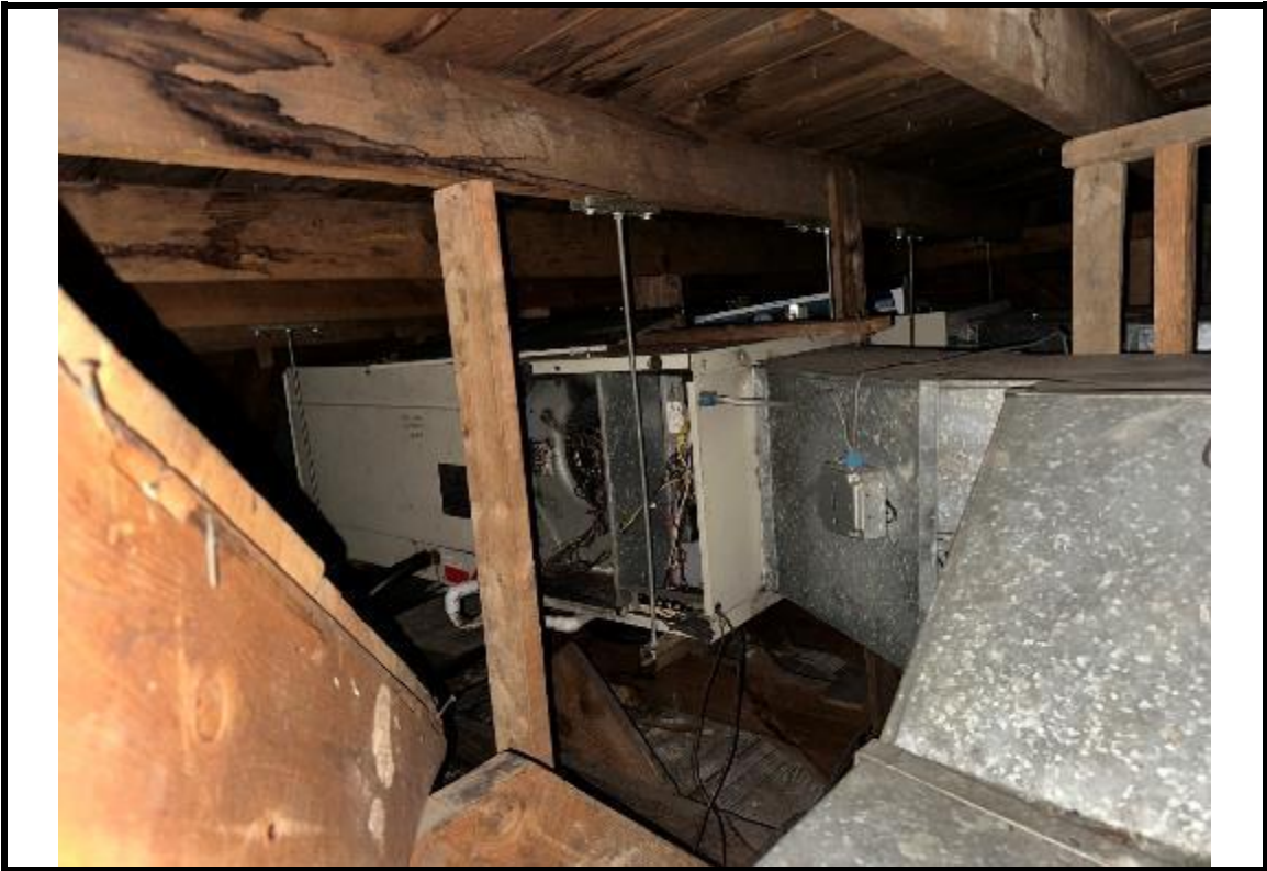
Photograph 55: Typical horizontal fan coil unit in attic space.
