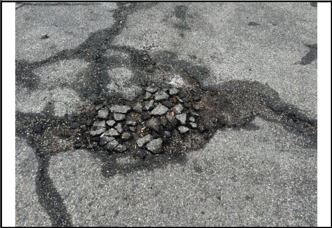
Photograph 7: Deteriorated asphalt pavement.
