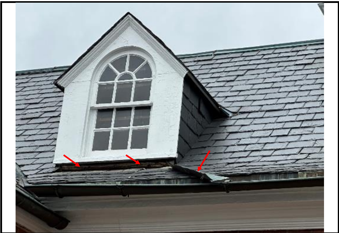
Photograph 34: Slate roof and dormer with displaced metal flashing. Note the loose and sagging gutter.
