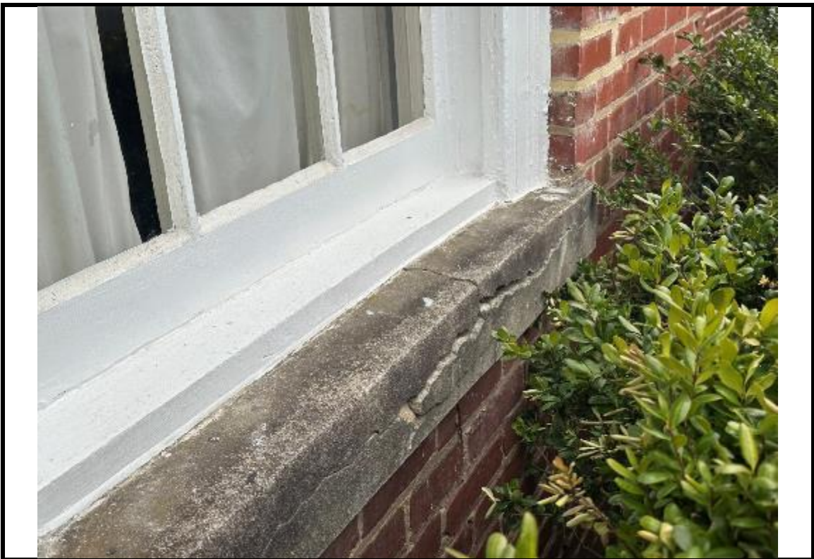
Photograph 32: Cracked stone window sill.
