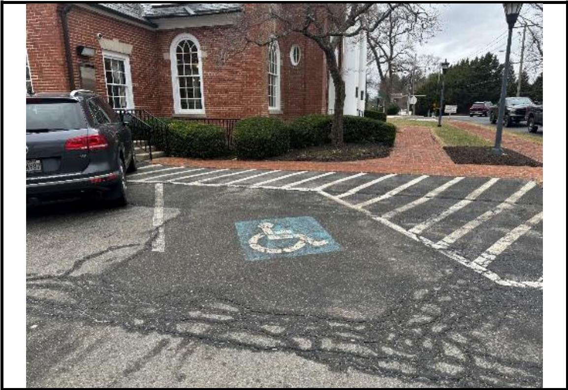
Photograph 5: Accessible parking space and access aisle.
