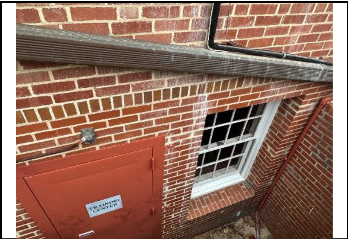
Photograph 28: Example of stained brick masonry.
