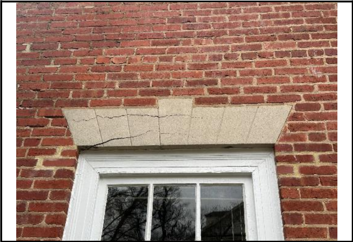
Photograph 29: Cracked cast stone above windows.
