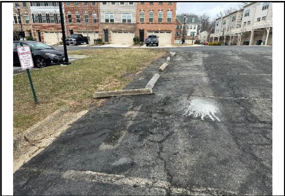
Photograph 4: South parking area. Note the displaced wheel stops.
