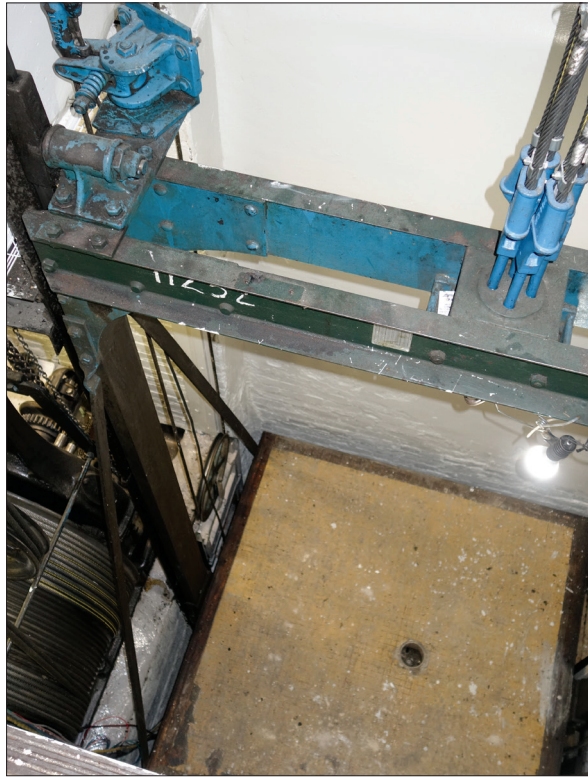
Fig. 7. Looking down the shaft at the original elevator-cab structure after the walls were dismantled, 2018. Components include the head beam with hoisting cable and vertical channels with diagonal straps supporting the original slung wood floor.
