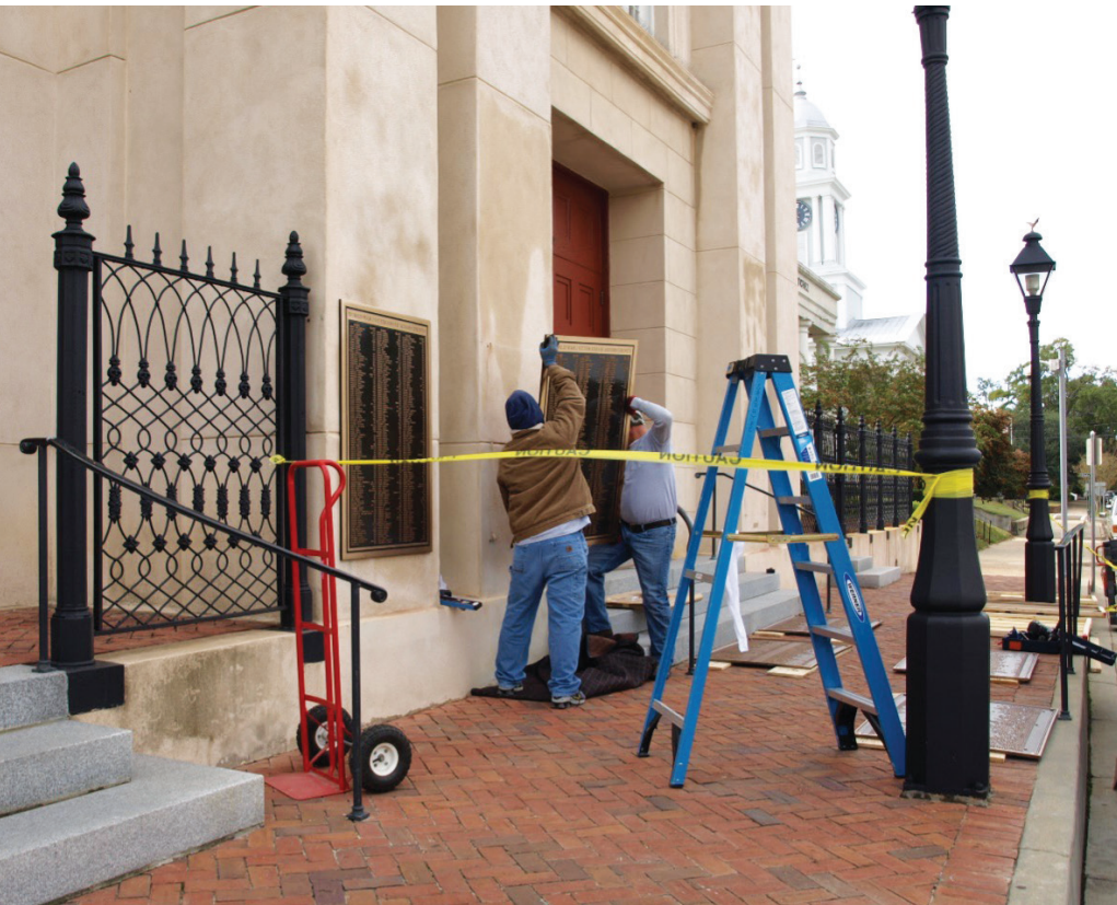
Fig. 6. Natchez Courthouse, Natchez, Mississippi, built in 1853 as the Natchez Institute School, showing the installation of the new informational plaques, rededicated in 2011. Courtesy of the U.S. General Services Administration, 2011.
