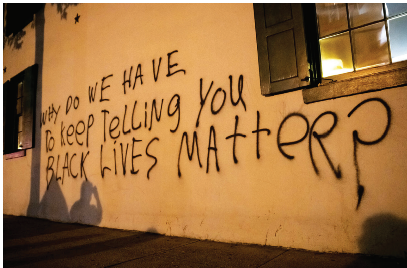
Fig. 12. Decatur House, Lafayette Square, Washington, D.C., built 1818–1819, with slave quarters added in 1821–1822, showing tagging as part of demonstrations in front of the White House to impress the lack of response to the Black Lives Matter movement. The house is a National Historic Landmark, owned by the National Trust for Historic Preservation. Photograph by Katherine Malone-France, 2020.
