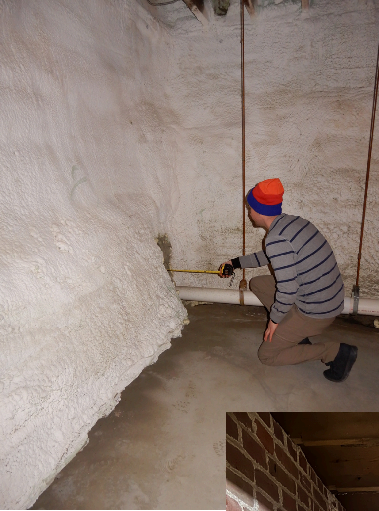
Gary Ogden measuring the displacement of spray insulation in the basement of the Old Labor Hall in Barre, Vermont.
