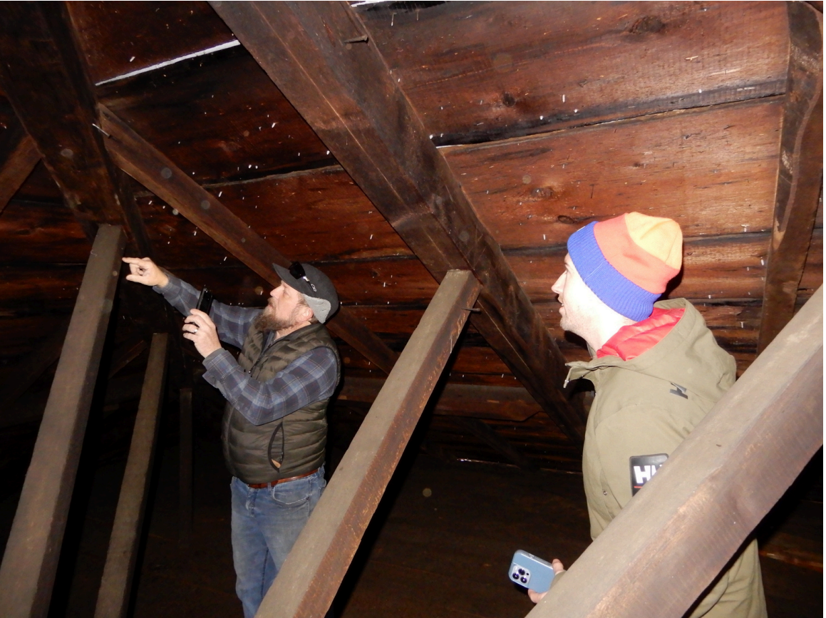
Gary Ogden and James Duggan of the Vermont SHPO discussing roof framing at Theron Boyd Homestead in Hartford, Vermont.
