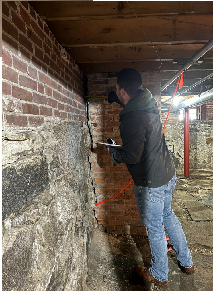
David Ribbans measuring the width of a crack at the Justin Morrill Homestead in Strafford, Vermont.
