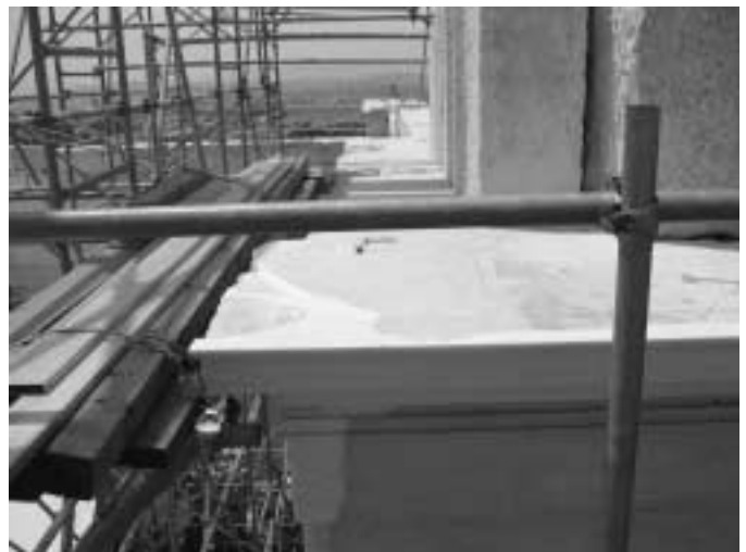
Fig. 2. Dutchmen inserted at the Propylaea, one of the monuments of the Athenian Acropolis, follow the exact geometry of the voids but are carved to the original exterior profile of the stonework, rather than the existing weathered profile. By this means the new material, although from the same marble quarry, is easily distinguishable from the original.
