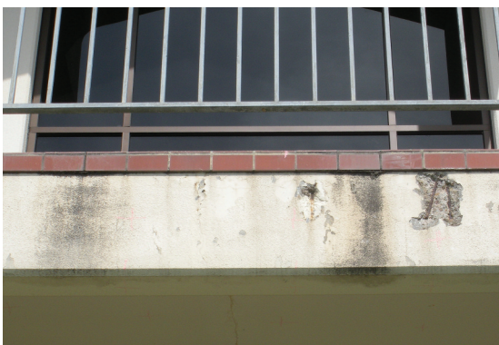
Fig. 3. College center building, west elevation, detail of edge of balcony slab. The structure has relatively low concrete cover, and the subsequent corrosion of the steel has caused spalling and has exposed reinforcing steel.
