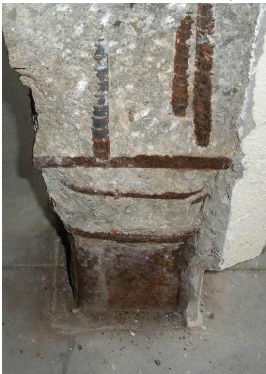
Fig. 2. College center building, west elevation. Detail of corrosion-related deterioration at column bases.
